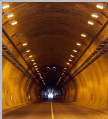
Tunnels and traffic stations
